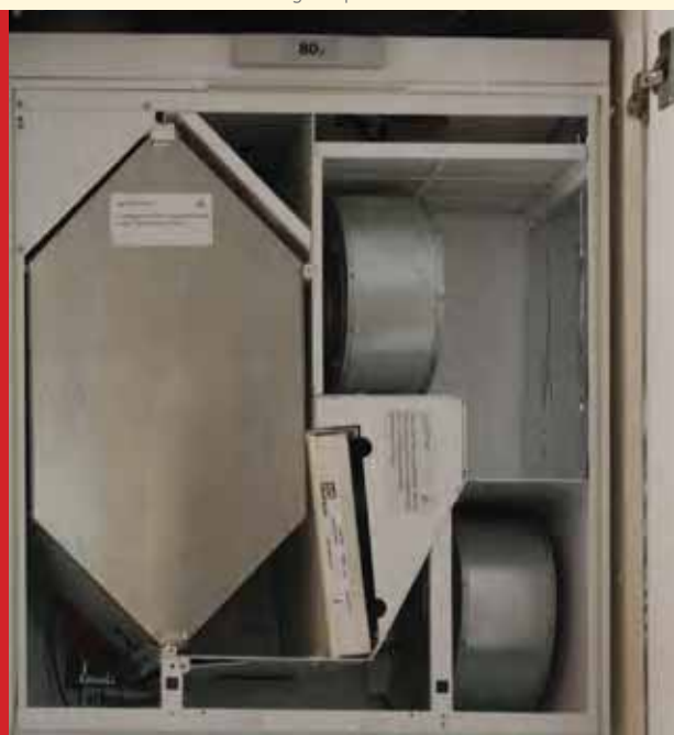
Ventilation unit with heat exchanger exposed
